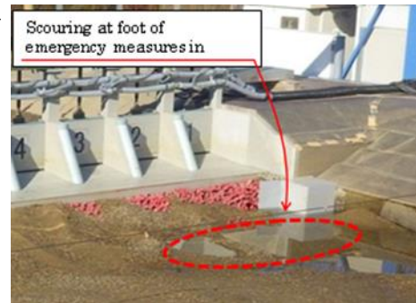
Figure 17. Stability test of emergency measures after design flood with fully equivalent gate operation
