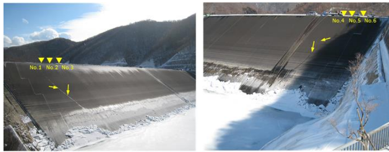
Figure 3. Asphalt facing of the Yashio dam right after the earthquake
