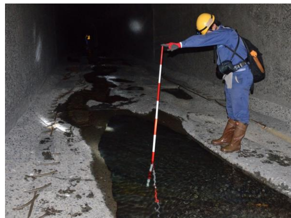
Figure 2. SBT invert abrasion (Asahi SBT)
