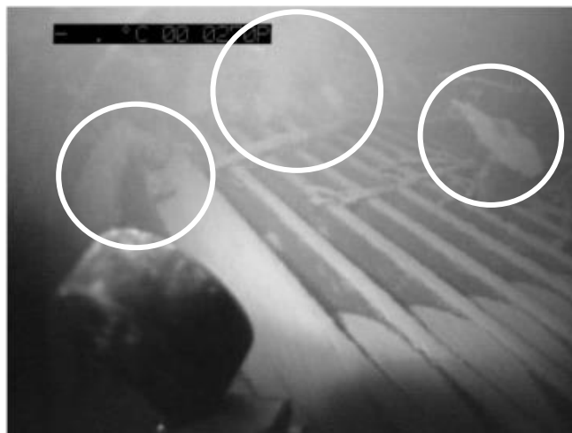
Figure 14. Sinkers above the bottom intake gate
