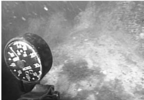
Figure 16. Sedimentation at the bottom intake side of the sediment retaining wall
