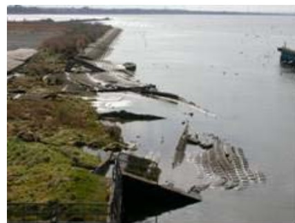
Photo 4. Damaged bank protection
