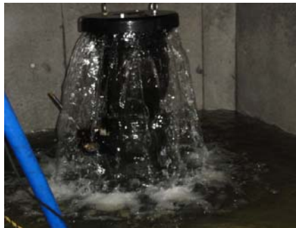
Photo 1. Damage of the air valve
