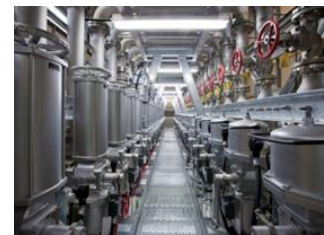
Figure 18. Air Control Unit Interior
