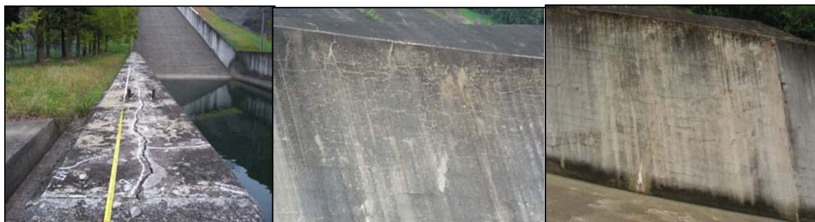
(a) Cracks on Top Surface of Training Wall
