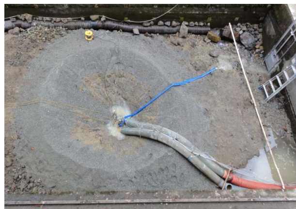
After sediment discharge
