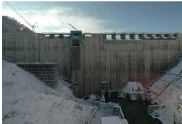
Figure 12. Progress of concrete placement for the Yubari Shuparo Dam in November 2011 (upstream surface).
