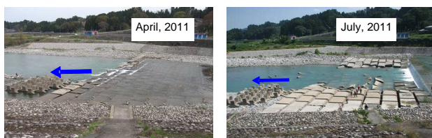
Figure 11. Destruction of the Ground Sill
