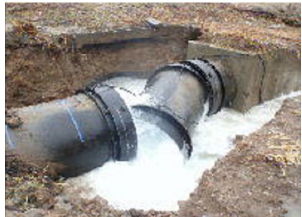
Figure 4. Damaged water pipe of the Sennan-Senen Wide-area Water Supply System of Miyagi prefecture
