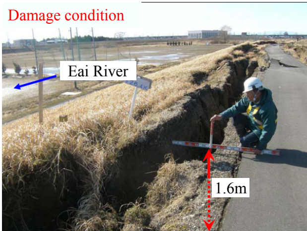
Figure 6. Damage of Eai River (Left bank: 25.9km + 20m to 26.9km)
