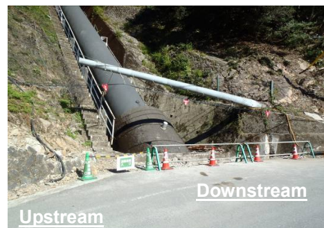
Figure 5. A leaning pole to upstream
