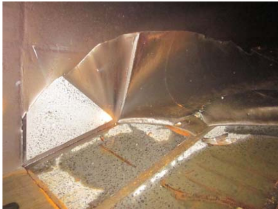
Figure 16. View of the damaged tunnel section lining with steel sheets
