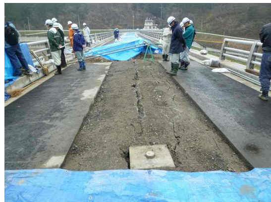
Figure 14. Cracking at crest at Koromokawa No.1 Dam (after removal of asphalt pavement)
