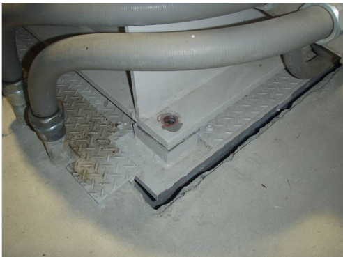
Figure 12. Shifting of hoist equipment and breaking of anchored bolts
