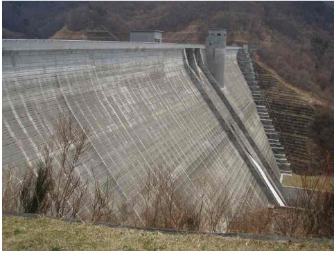
Figure 10. Takou Dam after the earthquake
