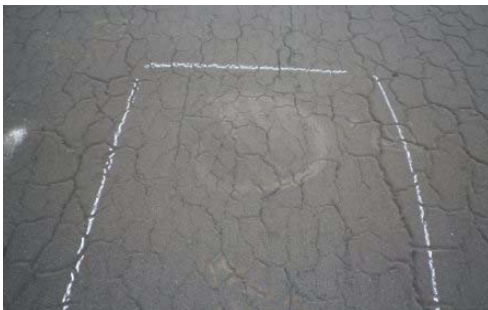
Figure 9. Blistering in the impervious layer
