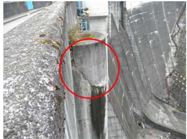
Fig.7. View of cracking of the downstream pier
