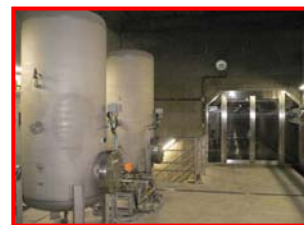
Figure 9. Onsite operation chamber
