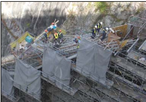
Figure 23. Construction of the training wall at the toe of the dam body (inclined portion)
