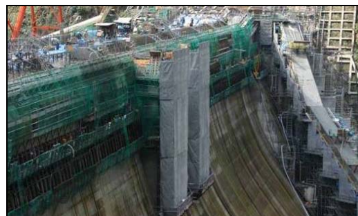
Figure 20. Construction of the deflector in the arc part of the overflow crest
