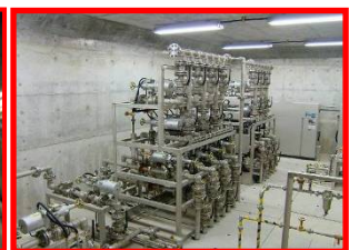
Figure 10. Valve control chamber
