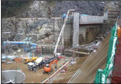
Figure 22. Construction of the training wall at the toe of the dam body (horizontal portion)
