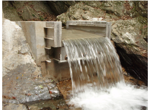
Figure 5 The accomplished conservation measurement. This measurement is a about 80cm waterfall with 30cm deep.
