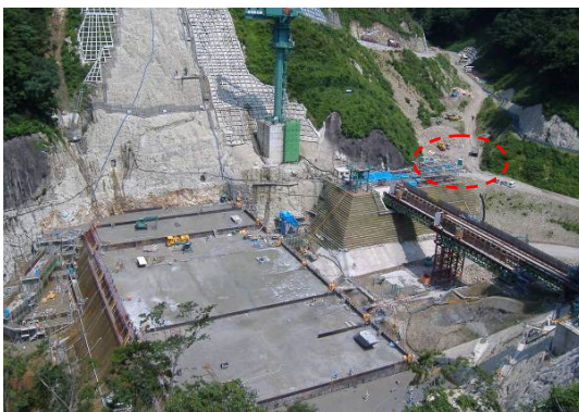
Figure 14. Intake tube assembly yard located within the operating radius of a tower crane.
