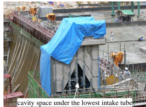
Figure 13. Installation situation of the lowest intake tube.
