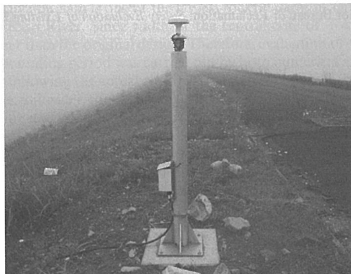
Figure 9. GPS installed on a rock-fill dam of EPDC.
