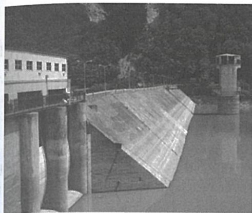
Photo 1. Concrete facing after the earthquake.
