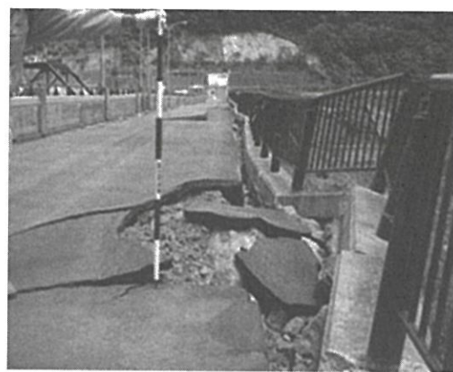
Photo 2. Deformation at the dam crest.
