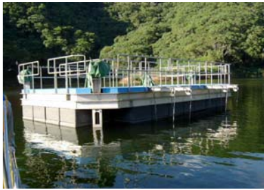
Fig.7 Deep layer aeration
