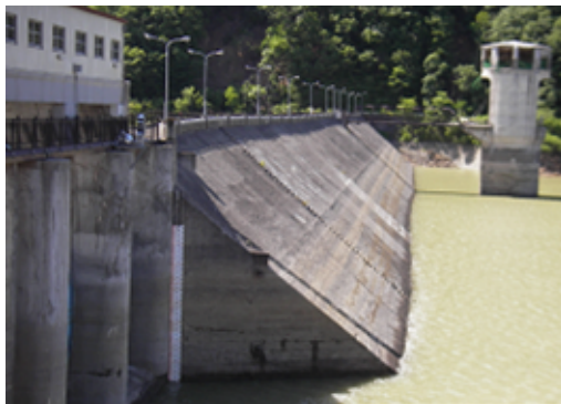
Fig. 2 Concrete faced upstream slope on which no damage was found at the Ishibuchi Dam June 15, 2008. [3]
