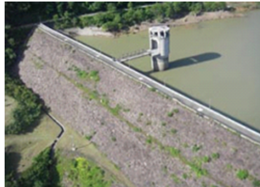
Fig. 3 Overview of the crest and downstream slope of the Ishibuchi Dam on June 15, 2008. [3]
