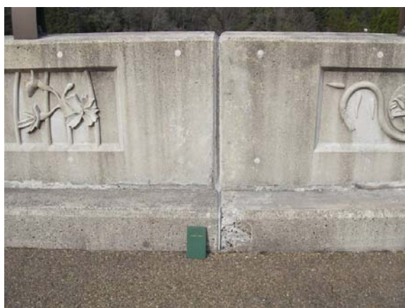
Photo. 3 Concrete chips between crest parapet joints on contraction joint J-8
