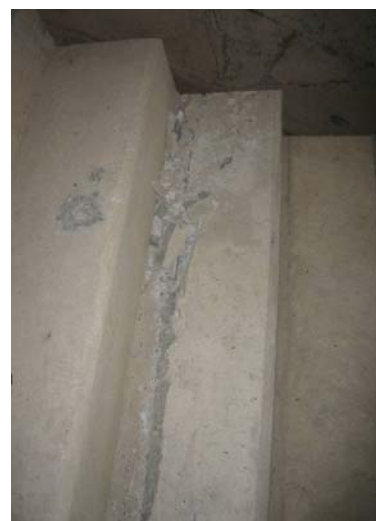
Photo. 4 Cracks in concrete steps along contraction joint J-8 in the gallery
