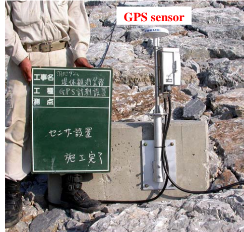
Fig.4 Close-up of an installed GPS sensor
