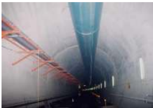
Photo 6 Belt Conveyor (left) and Blower Duct (right)
