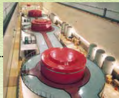
Generator of the Okutadami Power Station
