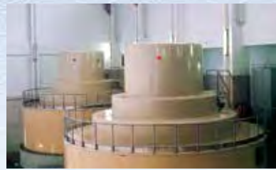
Generator of Kuromatagawa No.1 Power Station
