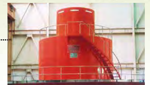
Generator No.1 of Ohtori Power Station
