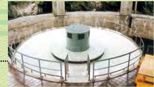
Generator of Ohtsumata Power Station
