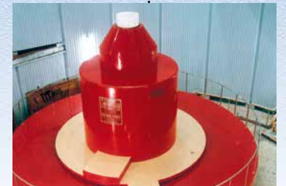
Generator of Kuromatagawa No.2 Power Station
