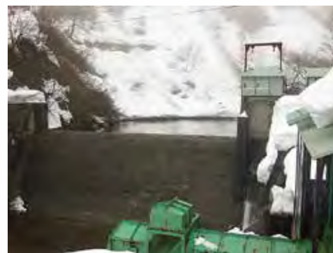
Hiraishi Water Intake Facility
