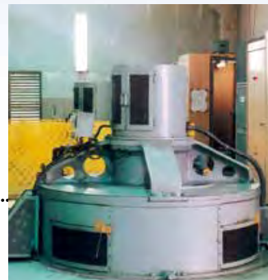
Generator of Suezawa Power Station
