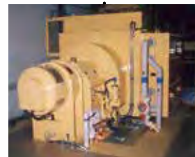
Generator of Okutadami Power Station (ecological flow)
