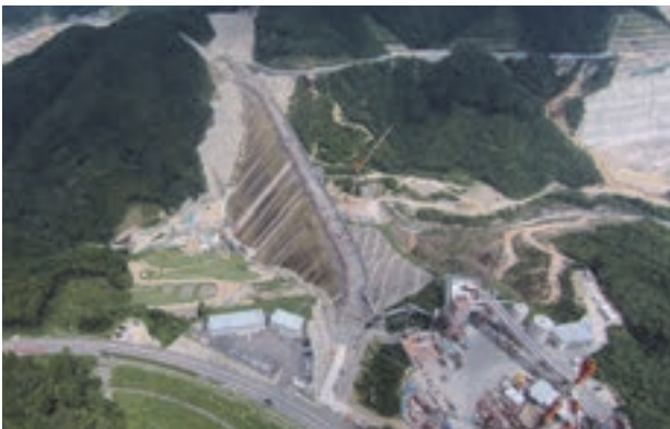
Figure 1. View of dam body placement (View of placement work on July 31, 2015, EL401.5m, 88 lifts)
