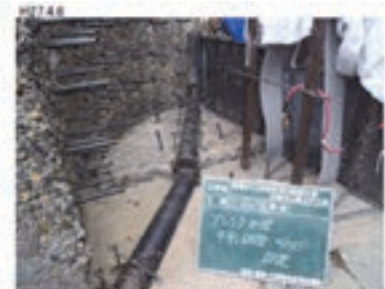
Crack break by the steel half pipe at EL193.3m
