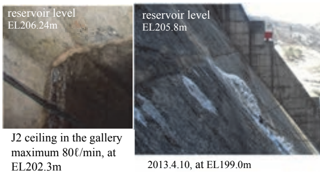
Figure 11. Water leakage situation through the J2 joint
