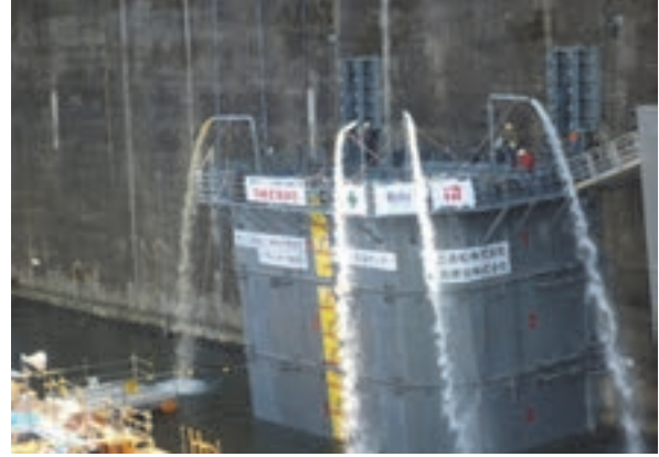
Figure 6. Drainage by pumps
