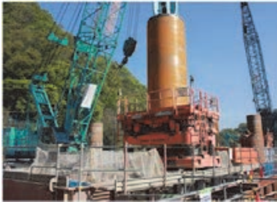
Figure 1. The conventional way of securing construction yard by installing a coffering structure (casing rotation excavation method)
