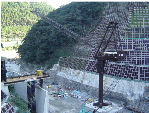
Photo 3. Low-brightness painting of tower crane
