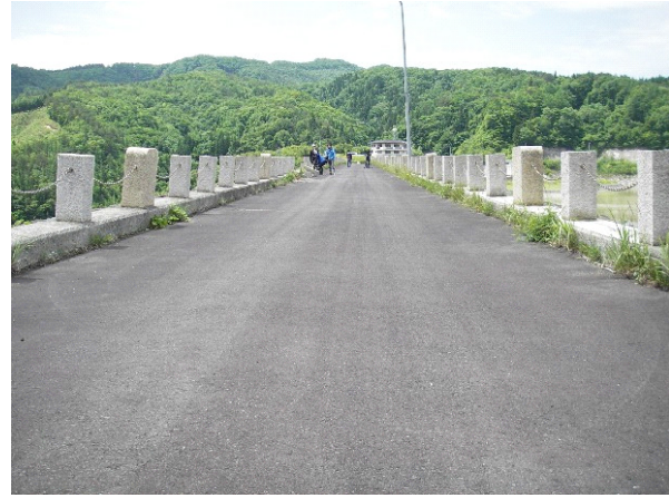
Photo.9 Few cracks in the crest pavement in spite of the dam body settlement (Aratozawa Dam) (Photographed by PWRI on June 16, 2008)
