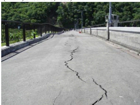
Photo.3 Cracks and waving of the crest pavement (Ishibuchi Dam) (Photographed by PWRI on June 15, 2008)
