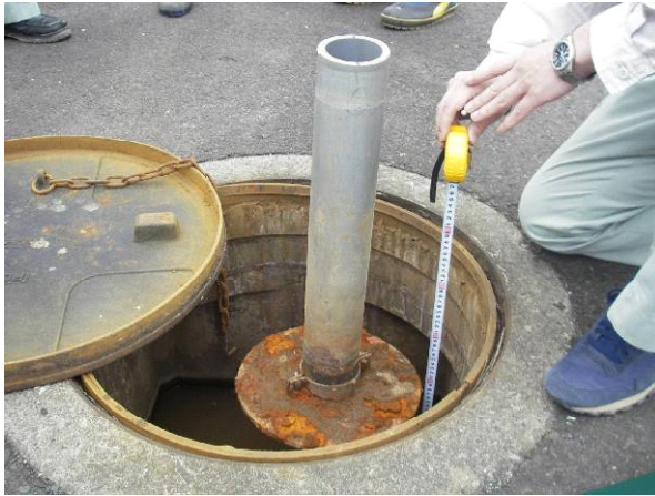
Photo.8 The pipe of a crossarm gauge protruded, as a result of the settlement of the dam body (Aratozawa Dam) (Photographed by PWRI on June 16, 2008)
