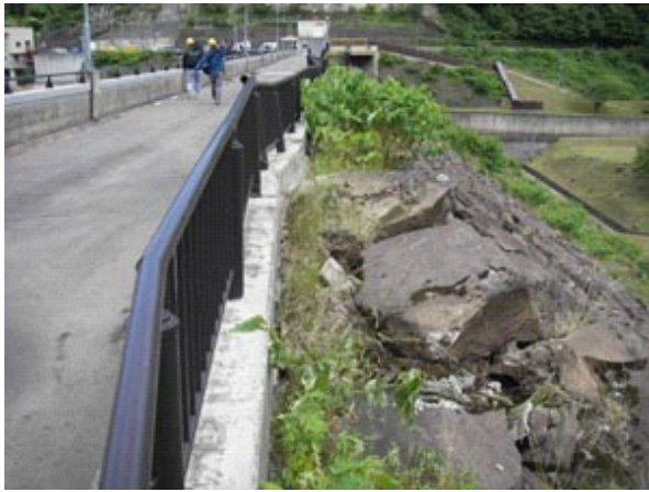
Photo.5 Projection of the riprap rocks around the top of the downstream slope (Ishibuchi Dam) (Photographed by PWRI on June 15, 2008)
