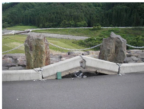
Photo.11 The damaged curbstone on the crest shoulder (Koda Dam) (Photographed by PWRI on June 16, 2008)
