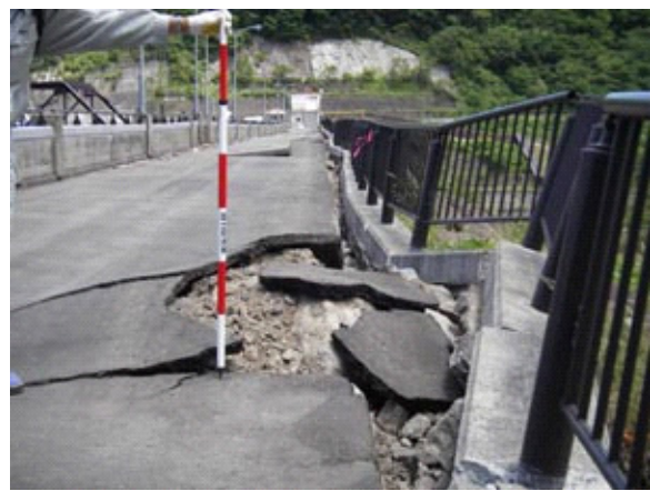
Photo.4 Gaps between the railing and pavement on the crest (Ishibuchi Dam) (Photographed by PWRI on June 15, 2008)
