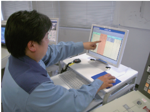
Fig.17 Remote Control System (Operation Room)
