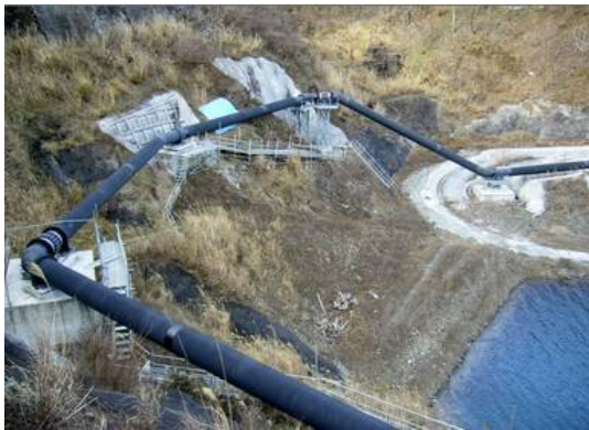
Fig.7 Steel Pipe Section (1)
