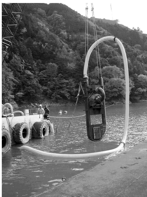
Photograph-2 Hydro-J Pipe
